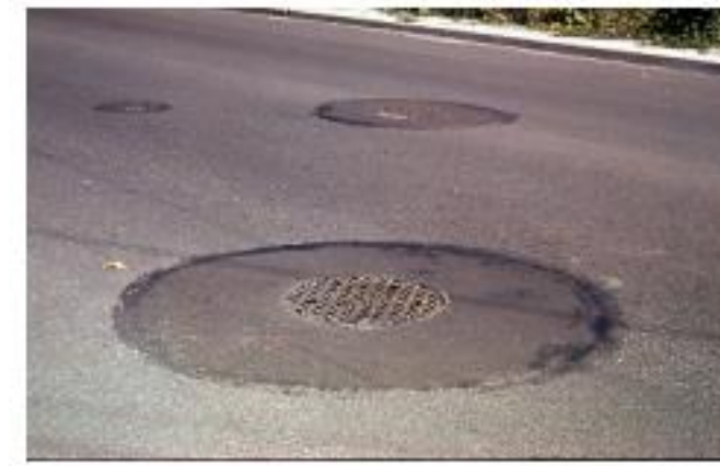
Figure 65. Manhole Iron Raised after Overlay
