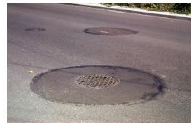
Figure 65. Manhole Iron Raised after Overlay
