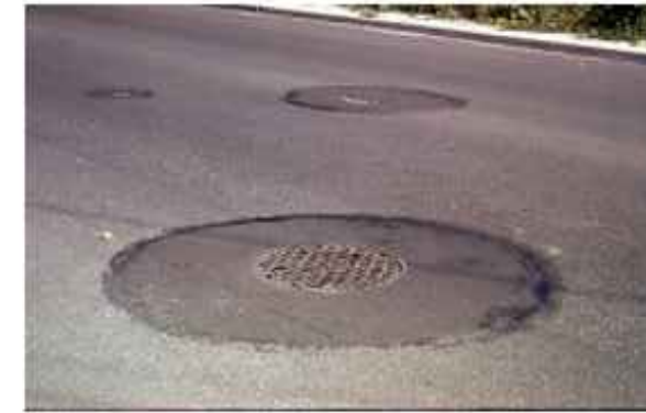
Figure 65. Manhole Iron Raised after Overlay
