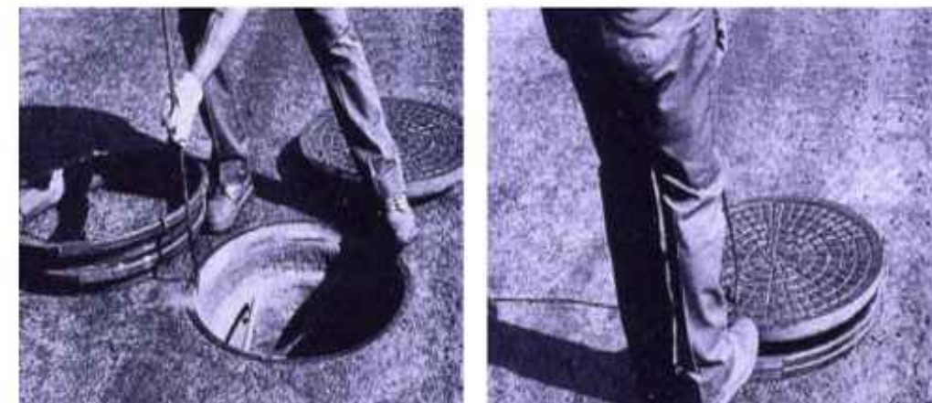
a. Clean Up Existing Manhole Ring & Cover b. Install Manhole Riser Ring
