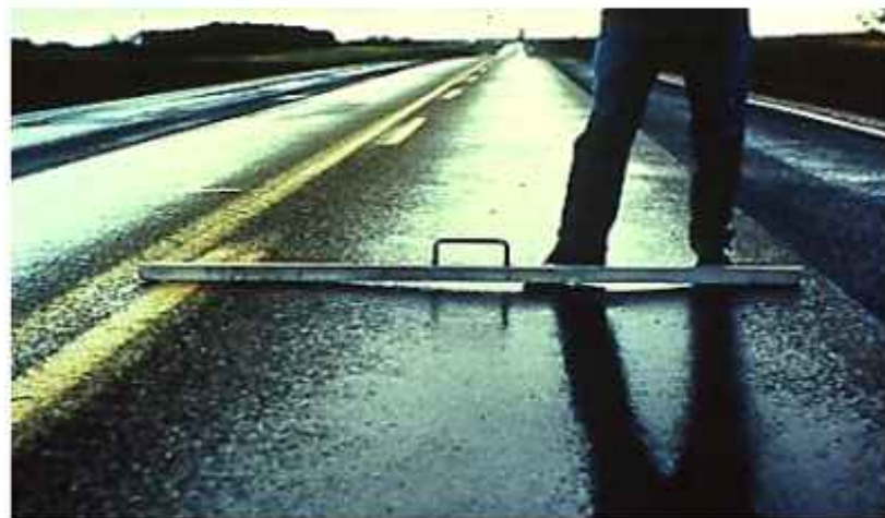
Figure 62. Rutting Requiring a Leveling Course Prior to Overlaying
